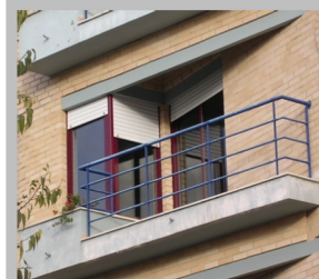
Dangerous distance between bars
